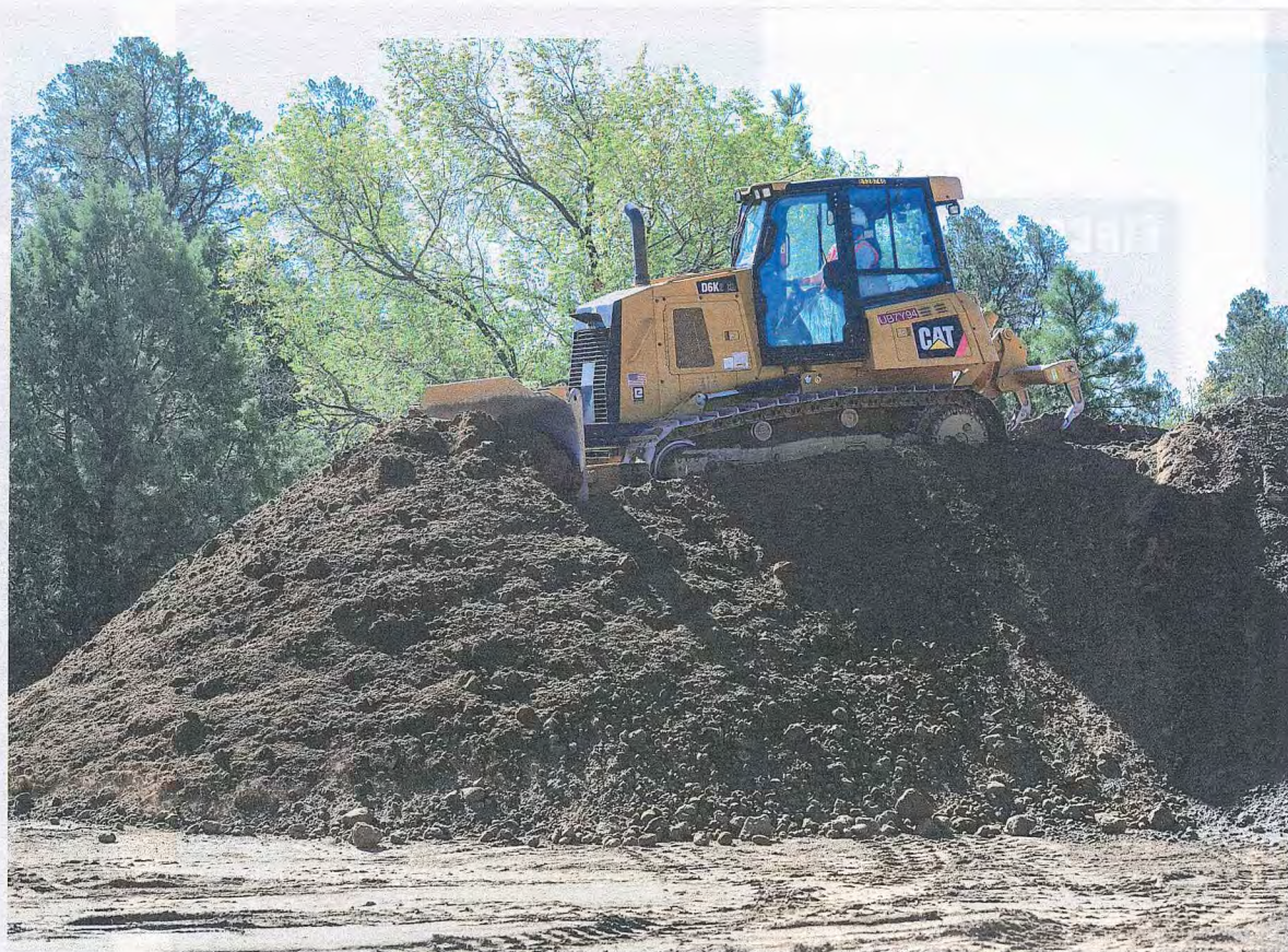
Lead remediation is expensive. A bulldozer moves the last pile of dirt with high lead content at the former Prescott Sportsmen's Club Shooting Range, April 18, 2017 in Prescott, Arizona. Cleanup costs approached $1.6 million. (Photo courtesy Les Stukenberg at The Daily Courier)
